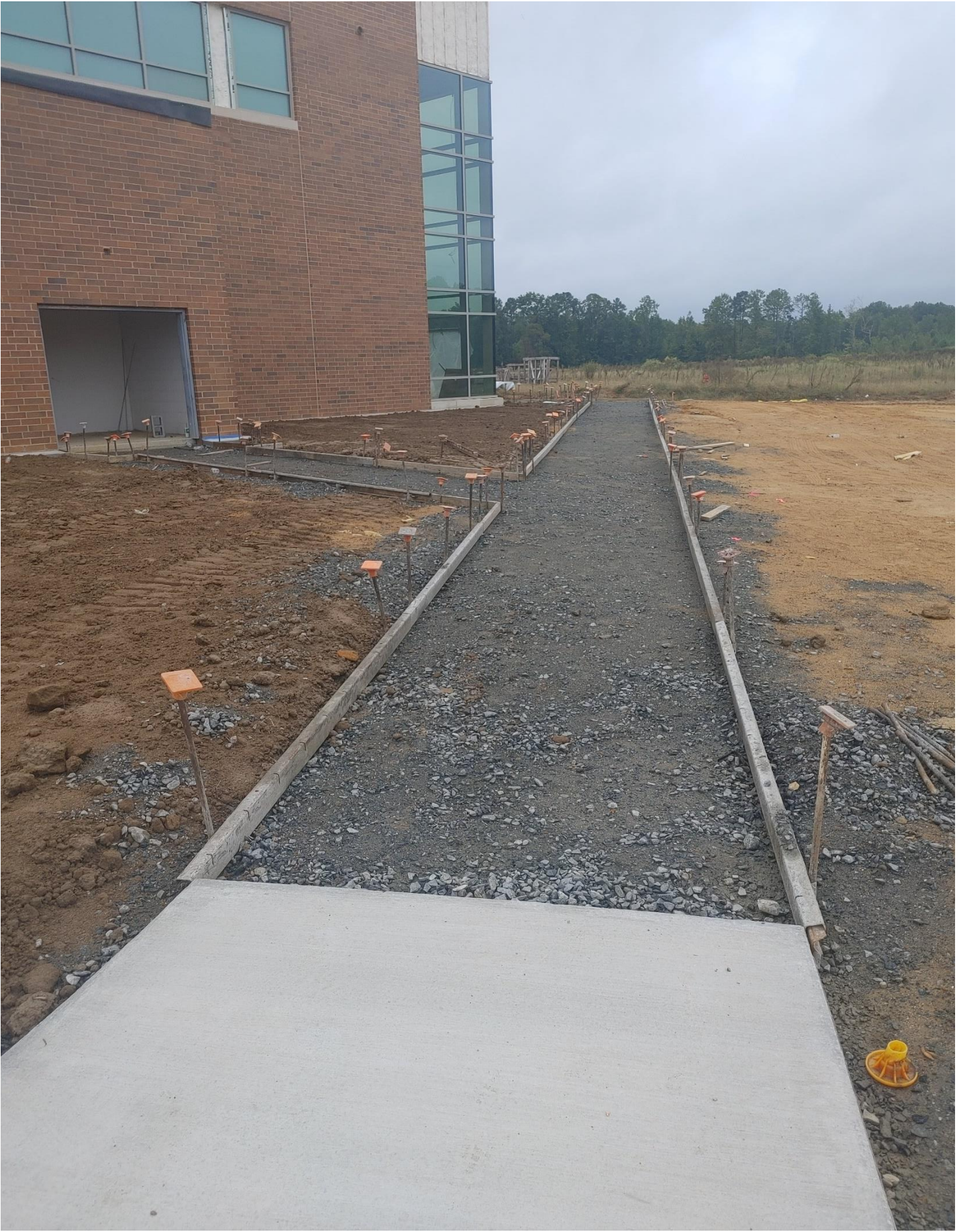
Photo 7 - Sidewalk prepped to be poured on the West side of Area E
