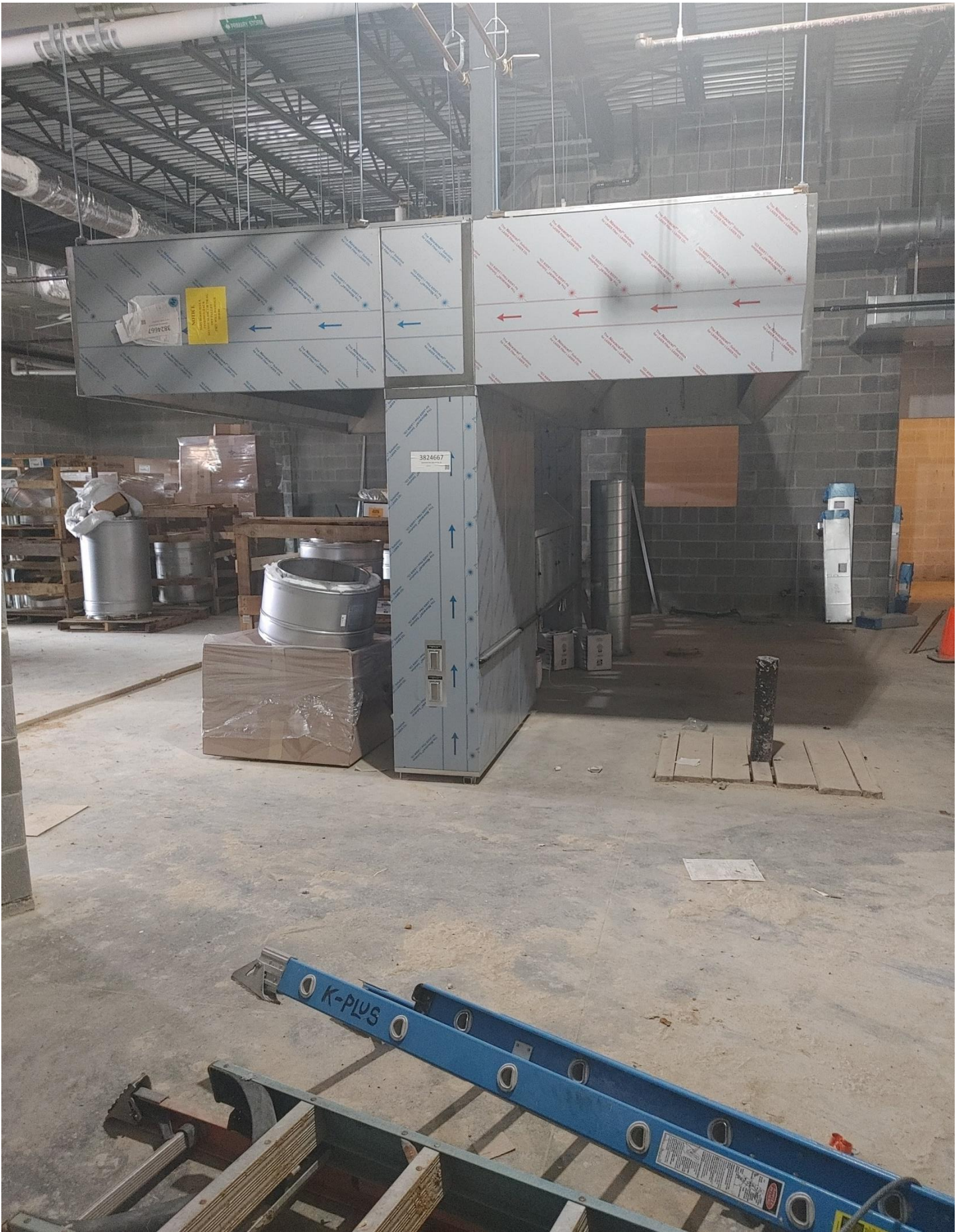
Photo 11 - The Kitchen Hood System has been installed
