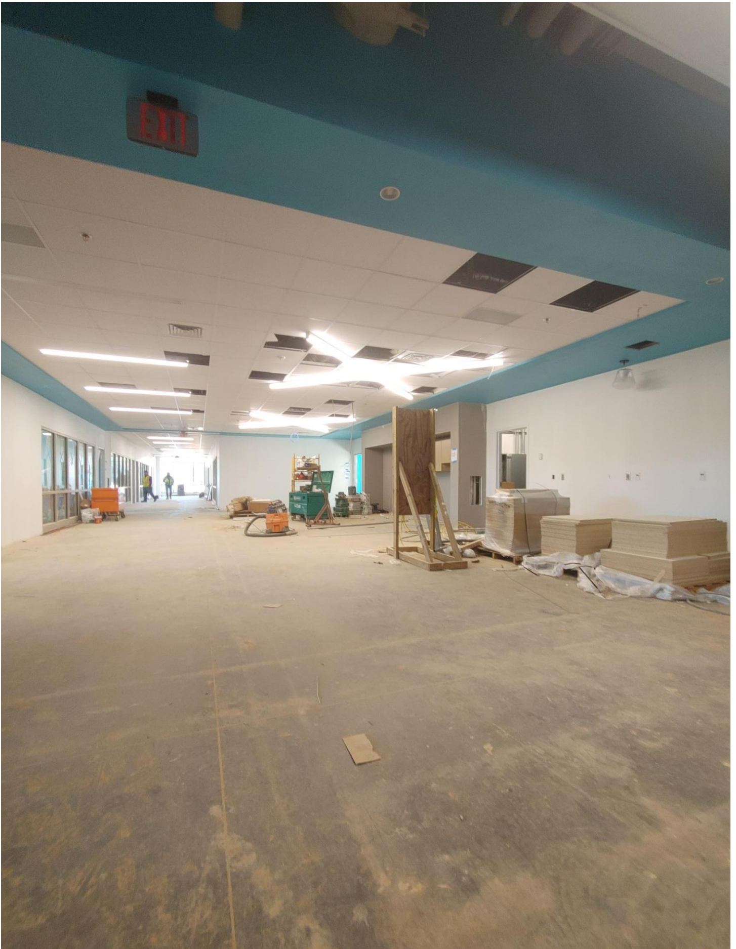
Photo 12 - LED Lights in Area A
