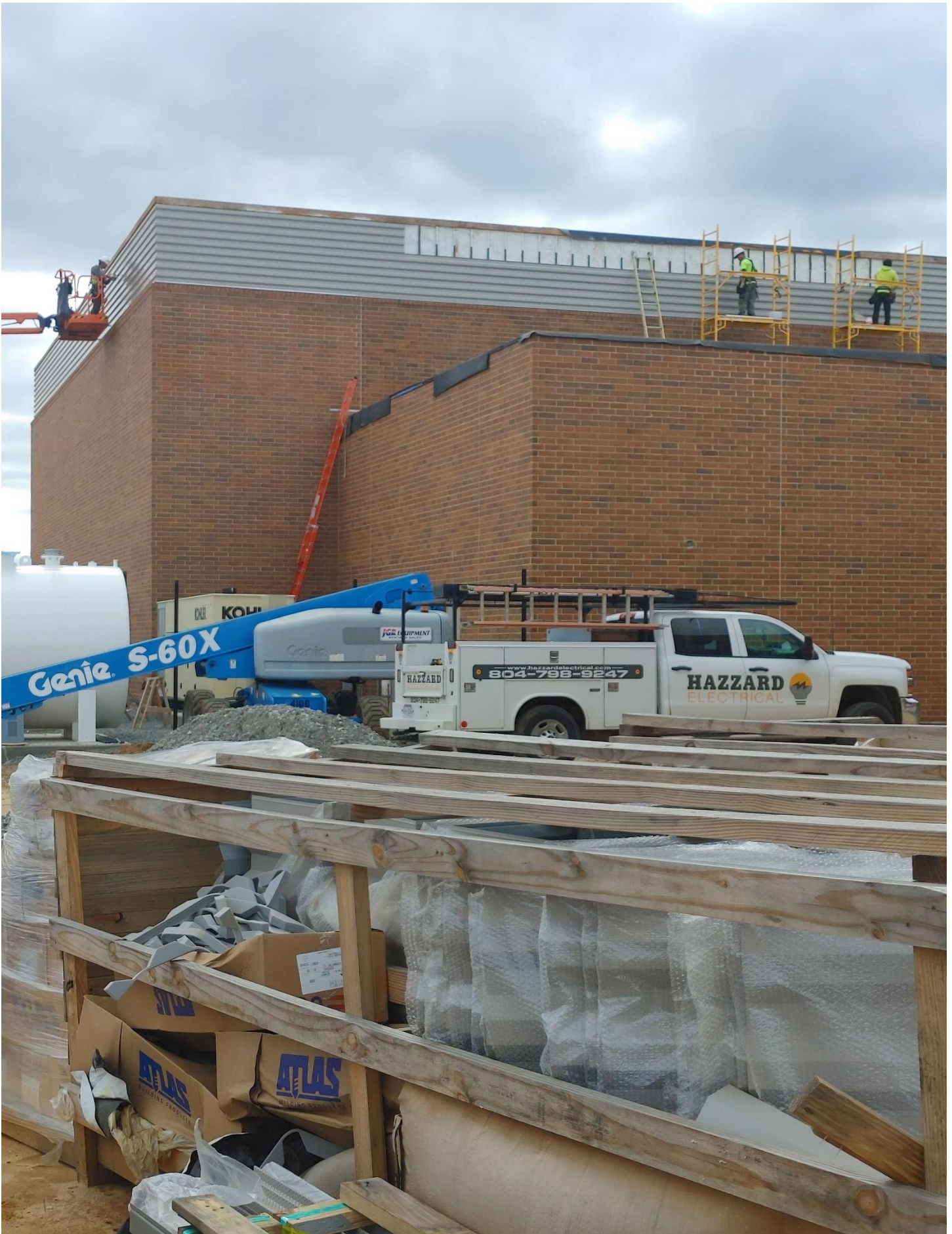
Photo 13 - Metal Panels are being installed on the East and North sides of Area D.
