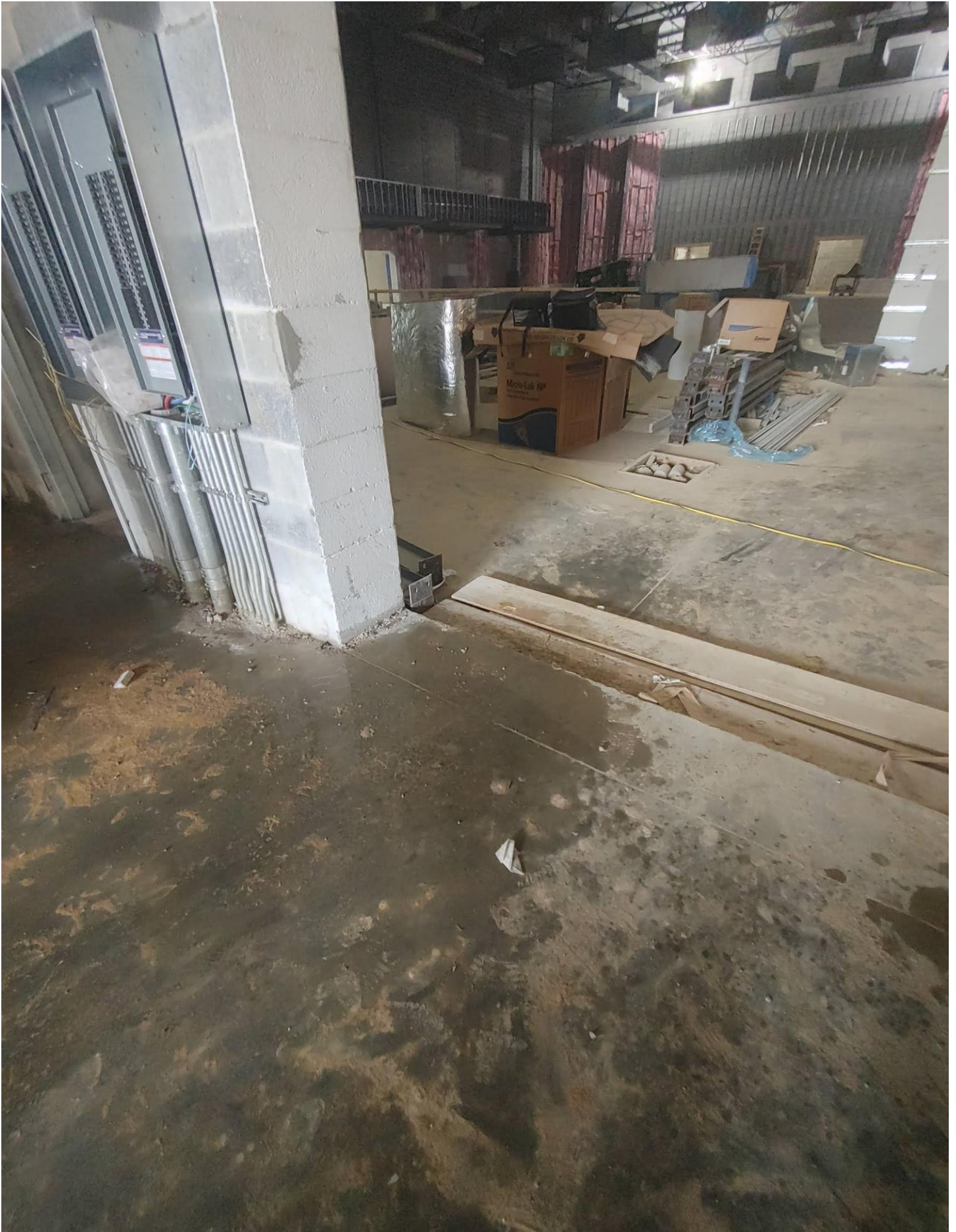
Photo 22 - Water dripping from Parapet wall above in Room D105
