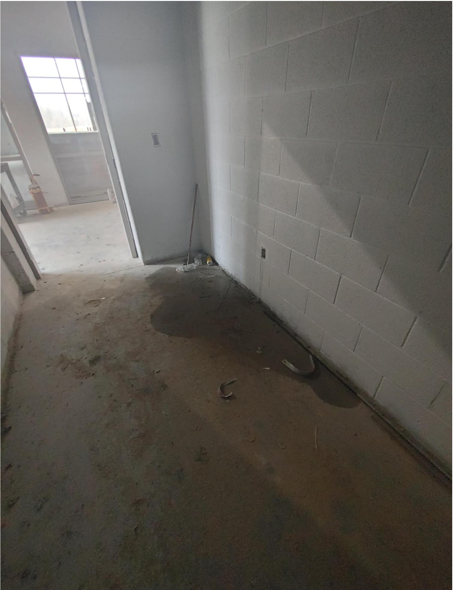
Photo 20 - Water leaking from parapet wall above in Corridor D13.
