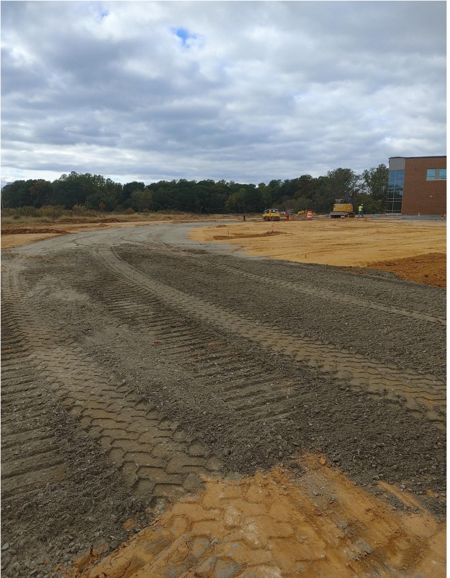
Photo 15 - Stone is being laid around the South side of the site for the access road
