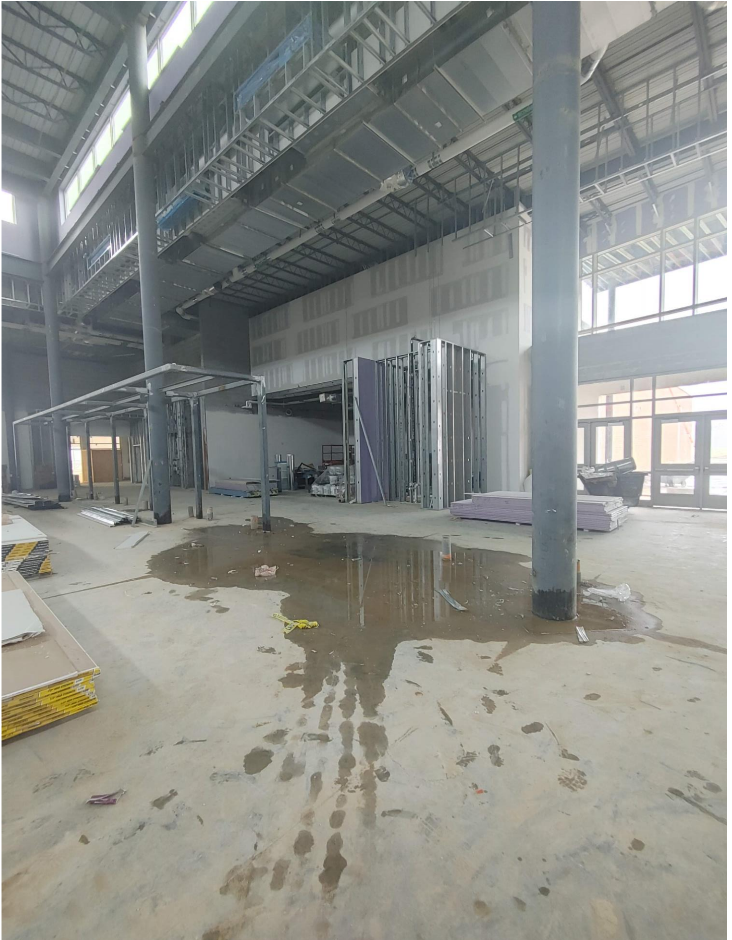
Photo 19 - Water leaking into Area C from windows above on the West side.
