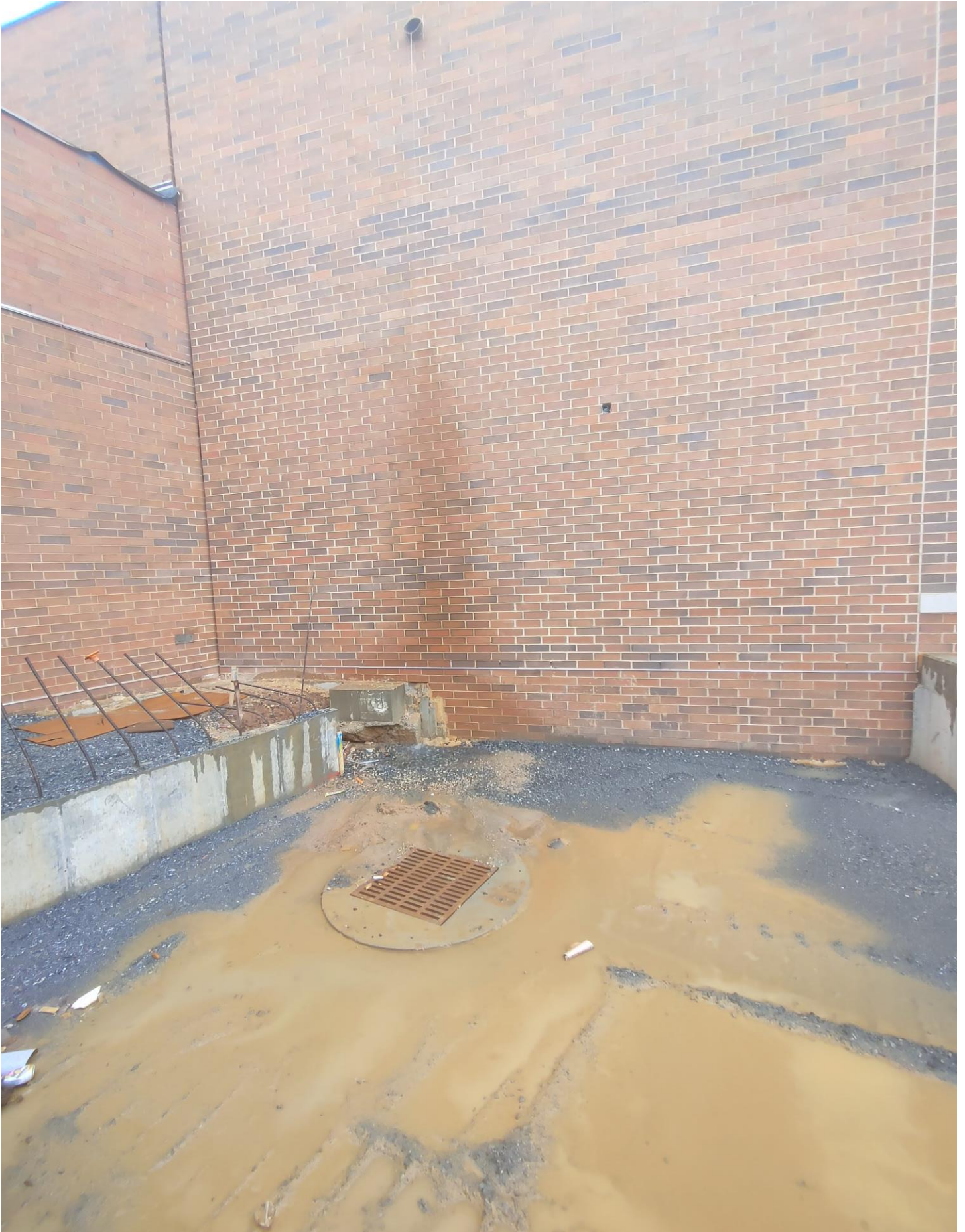
Photo 6 - Unprotected Drop Inlet in the Loading Dock Area allowing silt into the Storm Water Management System.
