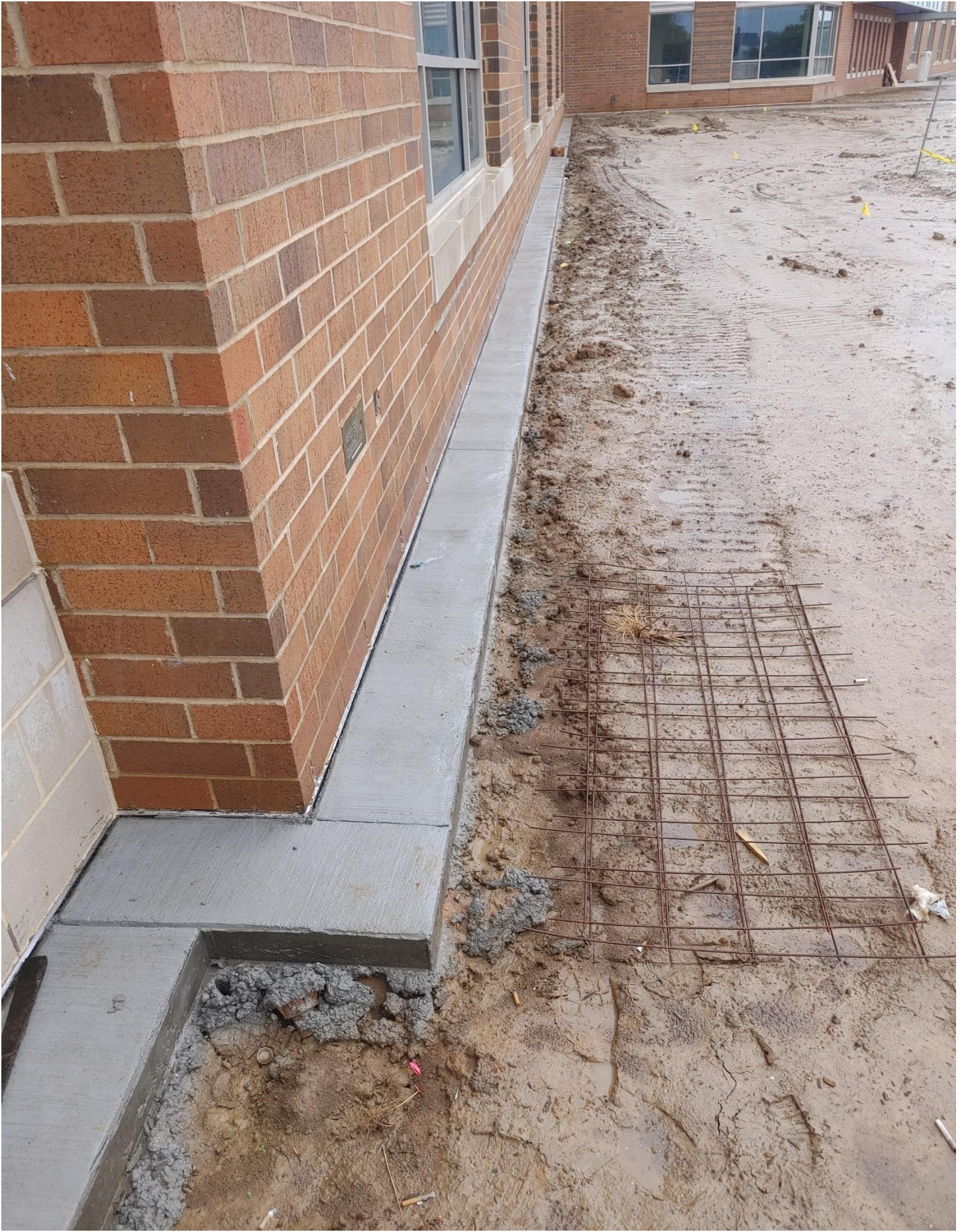
Photo 2 - The Mow Strip has been poured on the North side of Area A.
