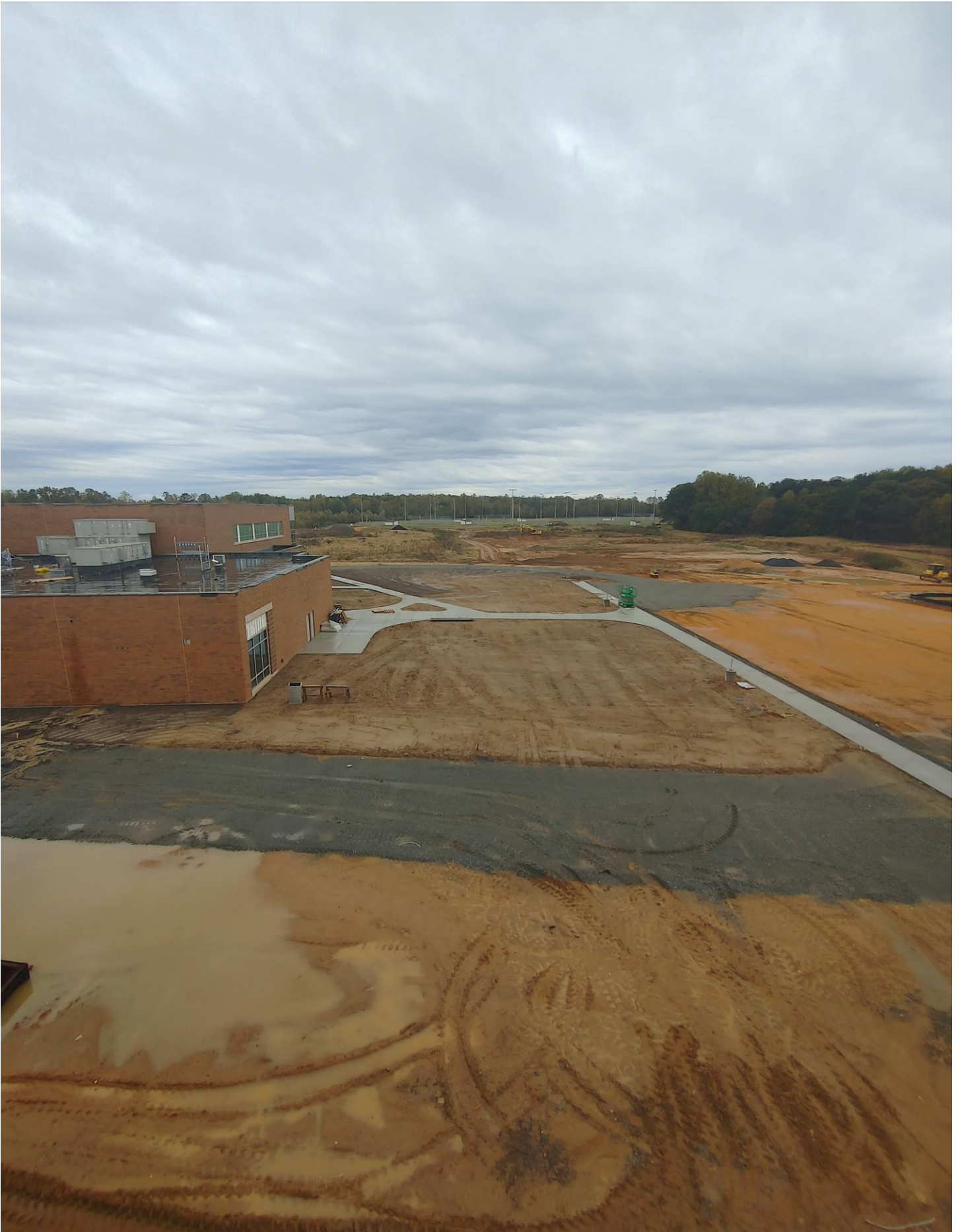
Photo 13 - View from the roof of the South West side of the site.
