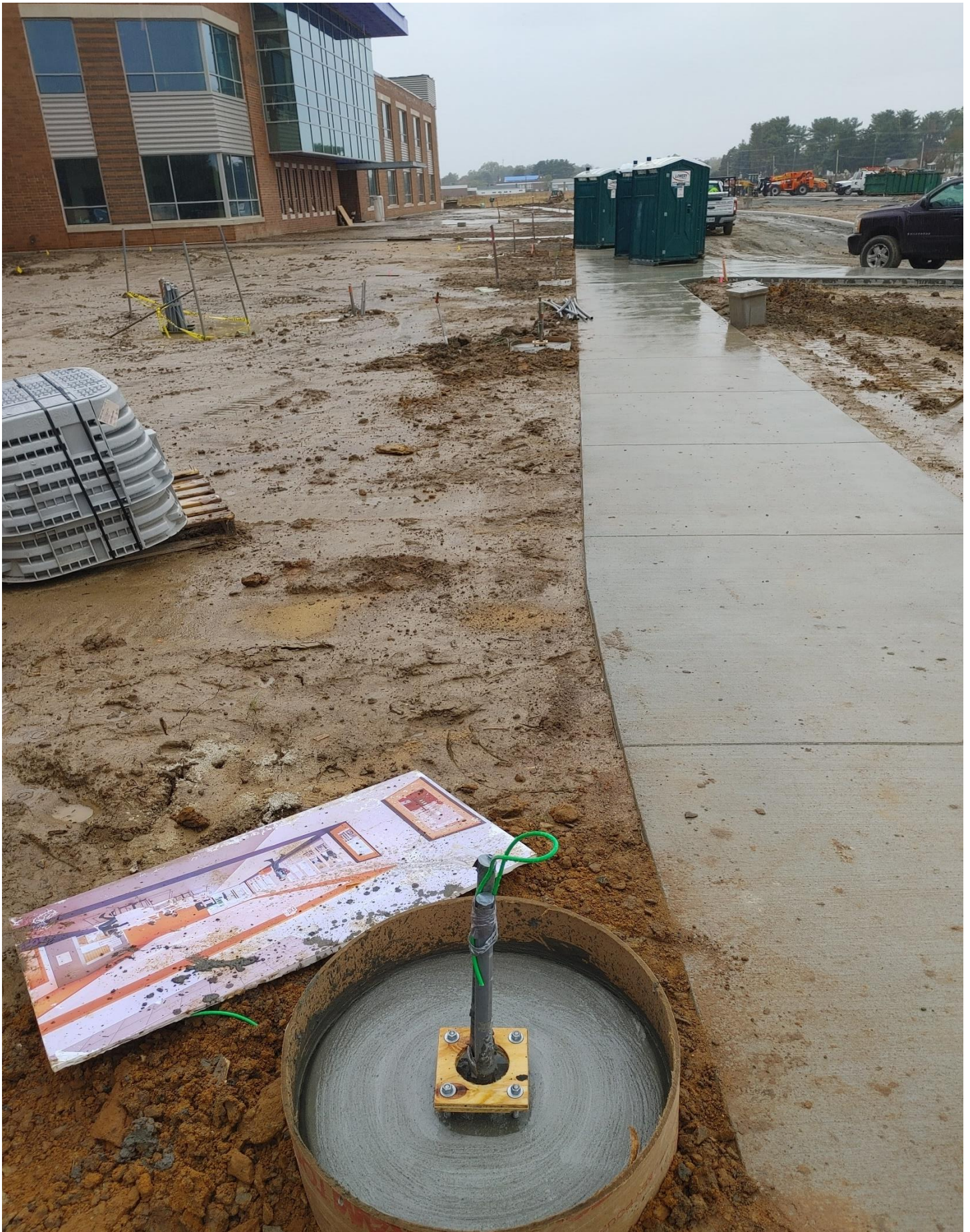
Photo 1 - They have begun to pour Light Poles Bases in front of the School.
