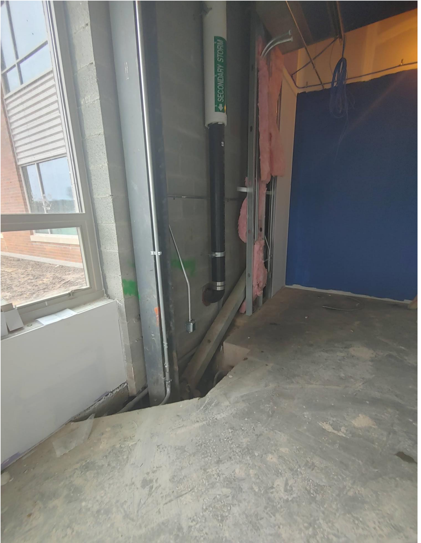
Photo 3 - Concrete has yet to be poured in the North East corner of the Administrative Office Area.
