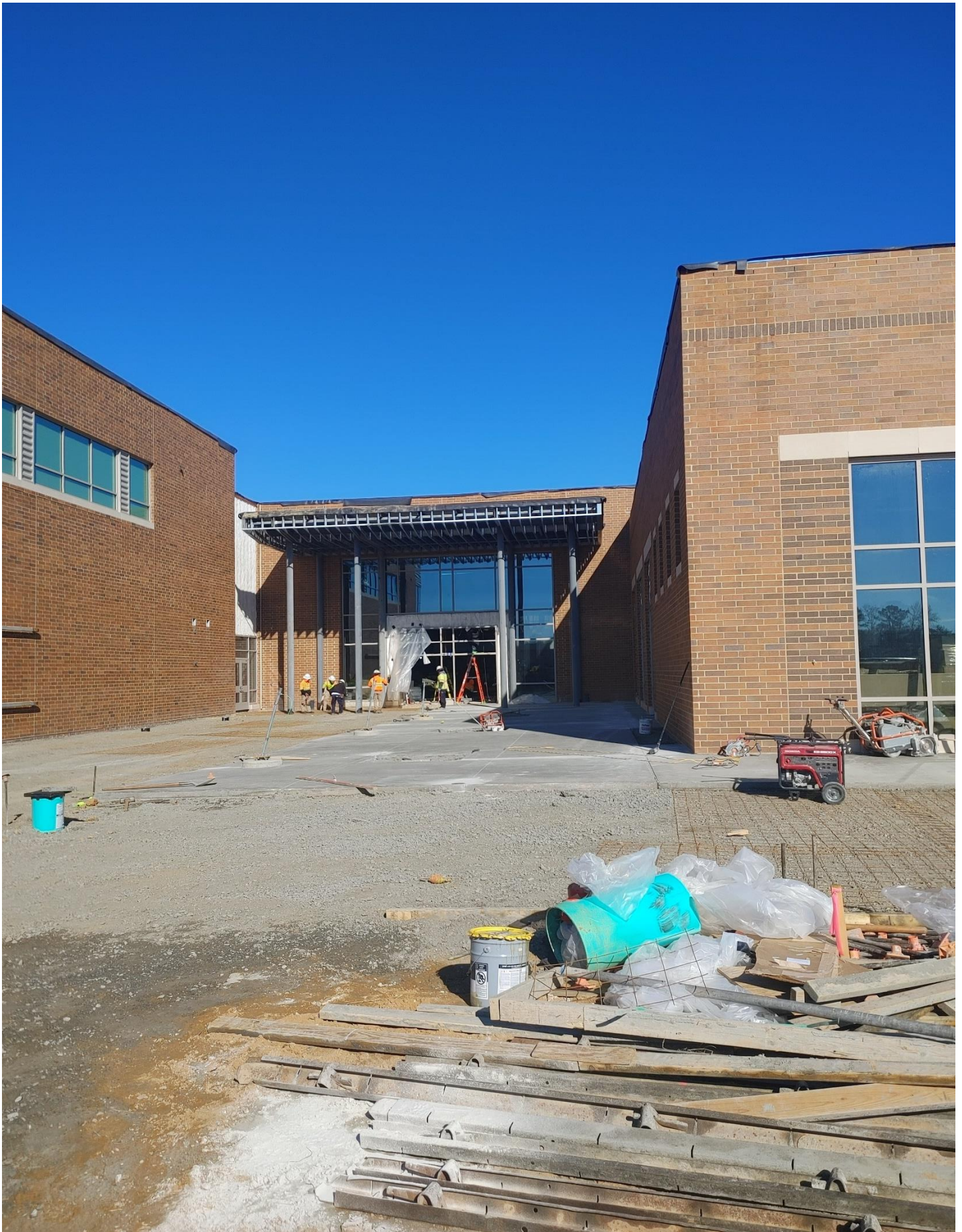
Photo 8 - Some of the Concrete has been poured on the South side of Area C. Remainder scheduled to be poured on Monday
