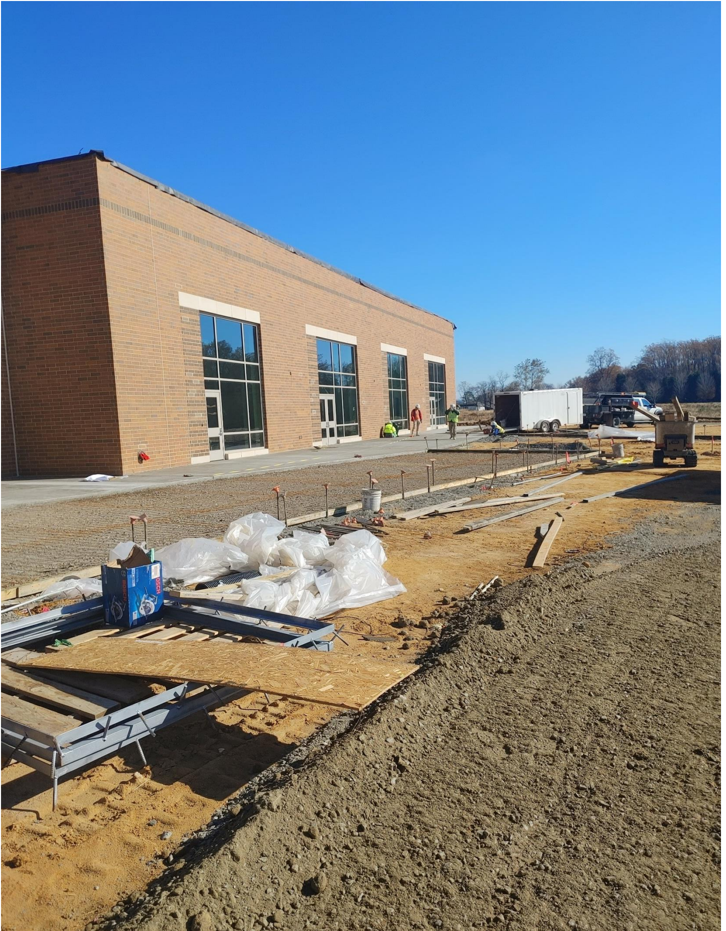
Photo 9 - Concrete forms are being erected on the South side of Area D.
