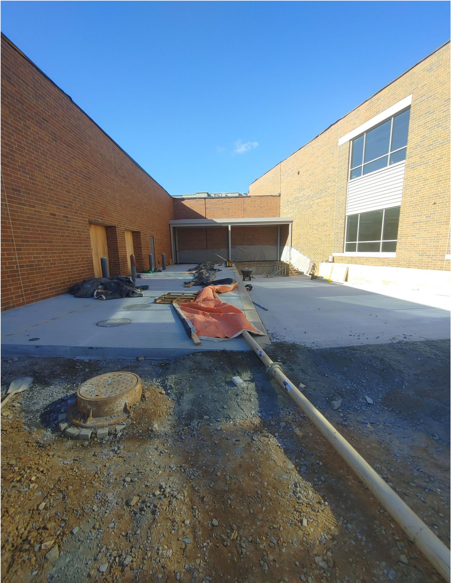
Photo 11 - Preparing to pour the remaining section of the Loading Dock and steps.
