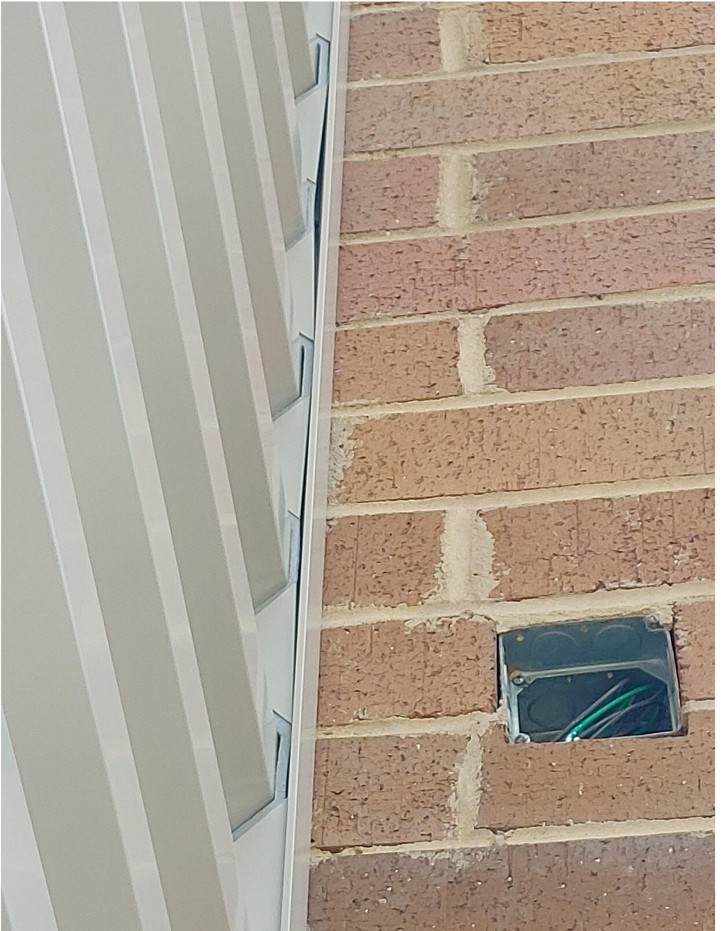
Photo 8 - Metal Channel areas to not be set properly on Stairwell #1
