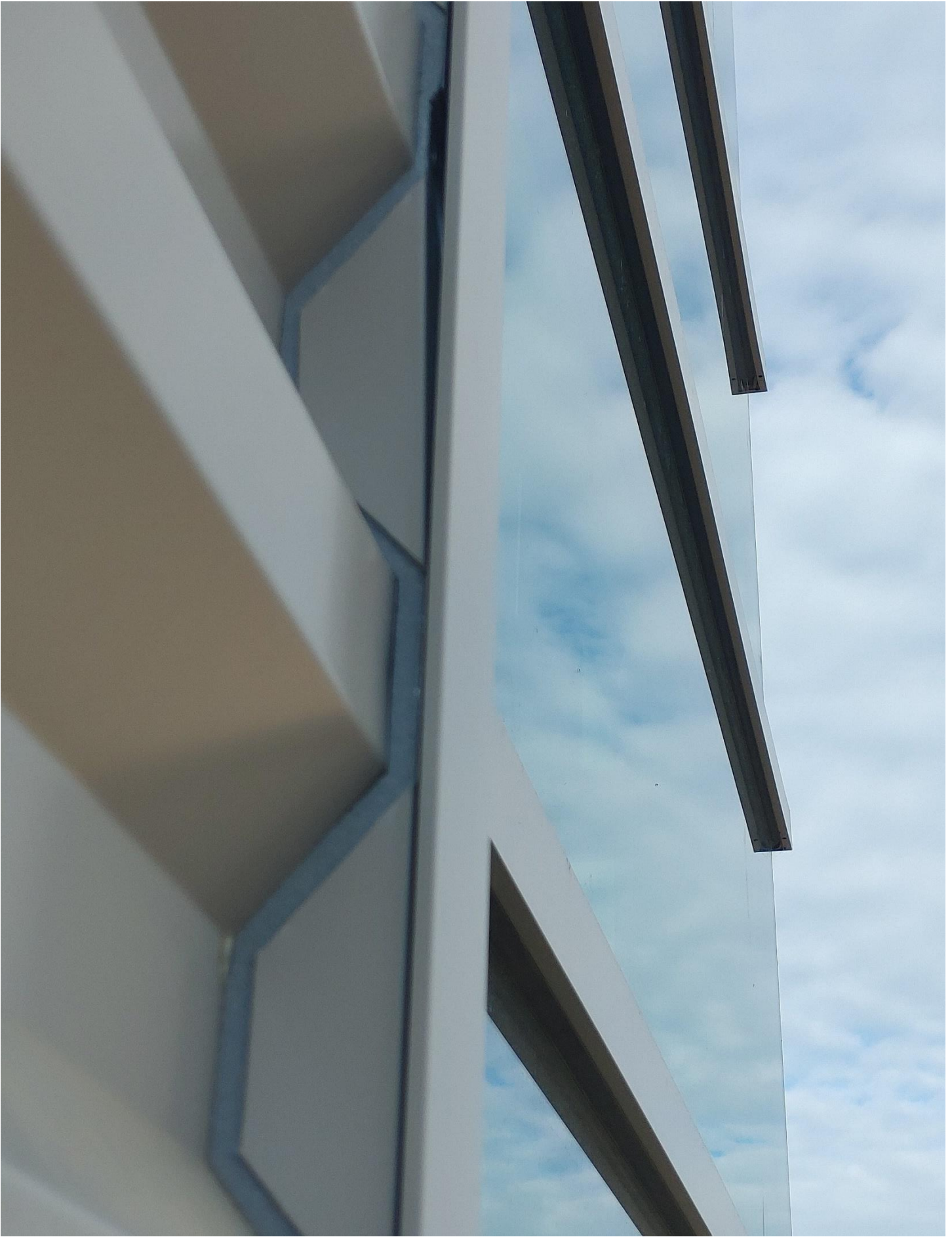
Photo 9 - Another area on Stairwell #1 where the Channel does not appear to be set properly
