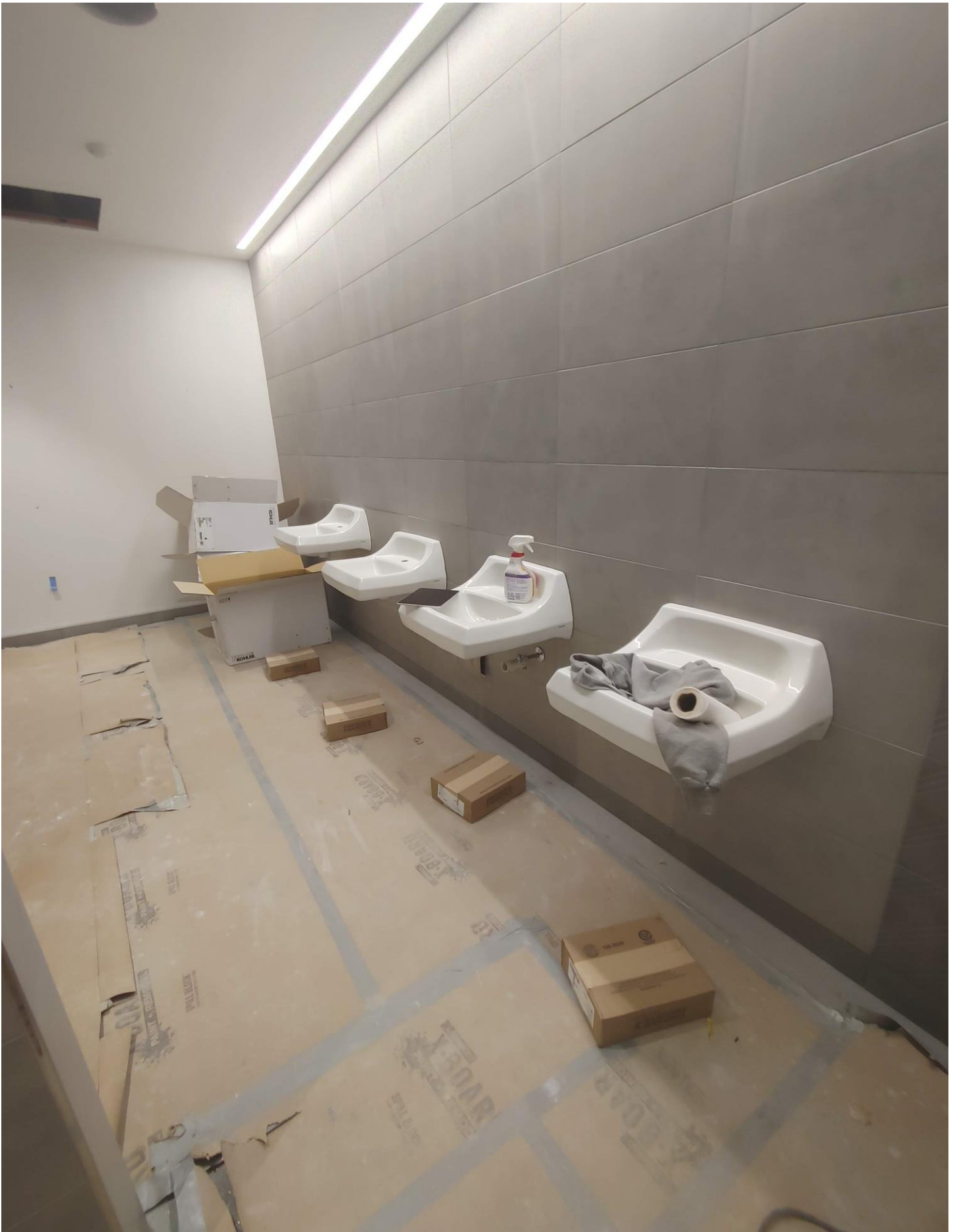
Photo 14 - Fixtures are being set on the first floor of Area A in A116.
