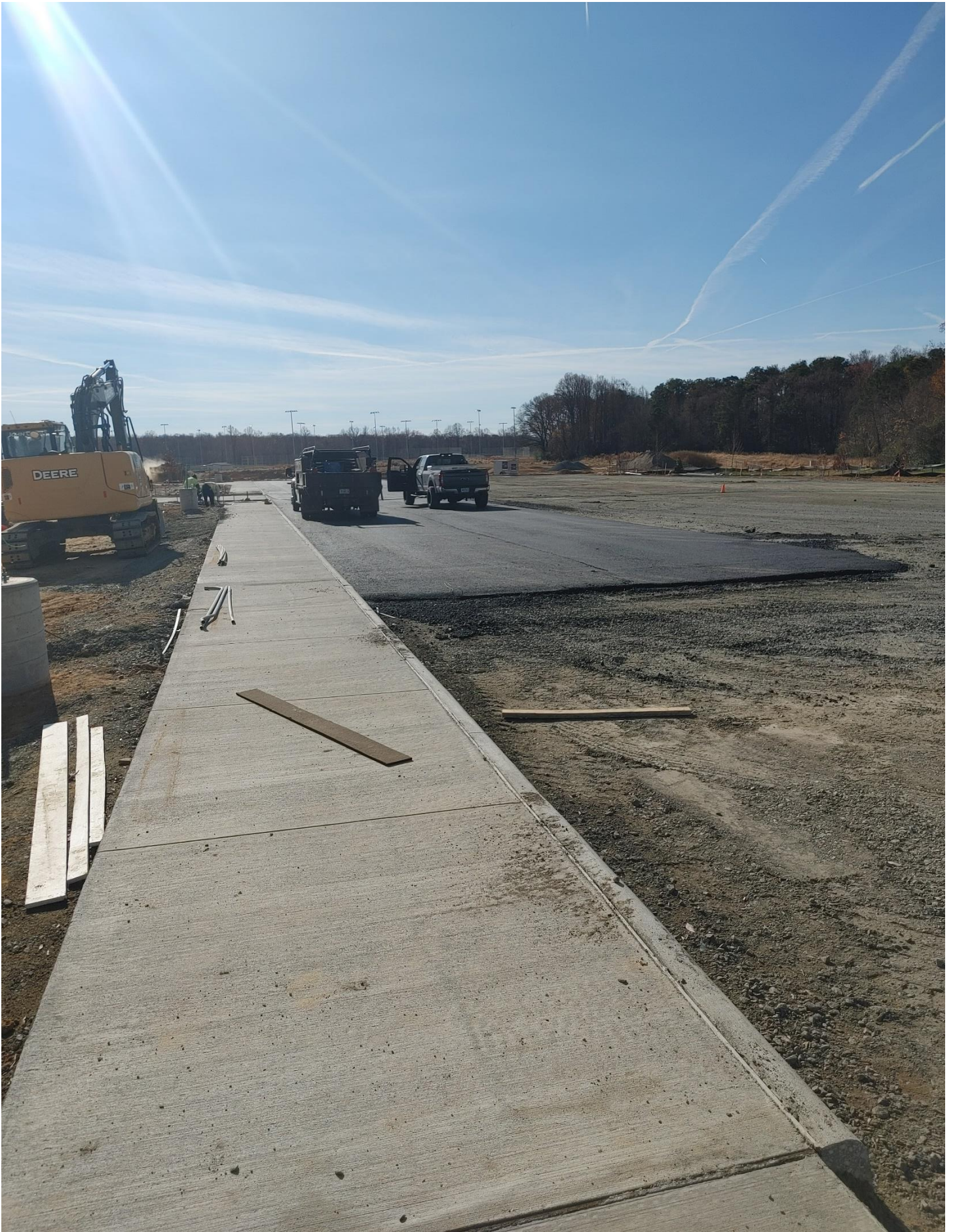
Photo 1 - Base layer of Asphalt is being laid in the Bus Loop area
