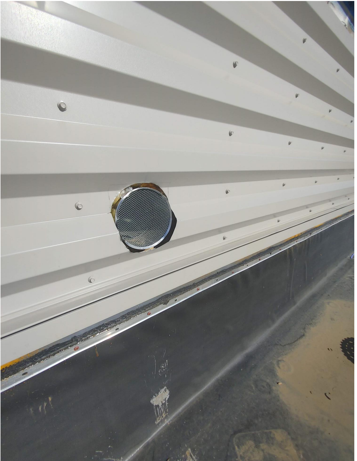
Photo 12 - Vent cut out on the South side of the high roof of Area A. Needs proper flashing.
