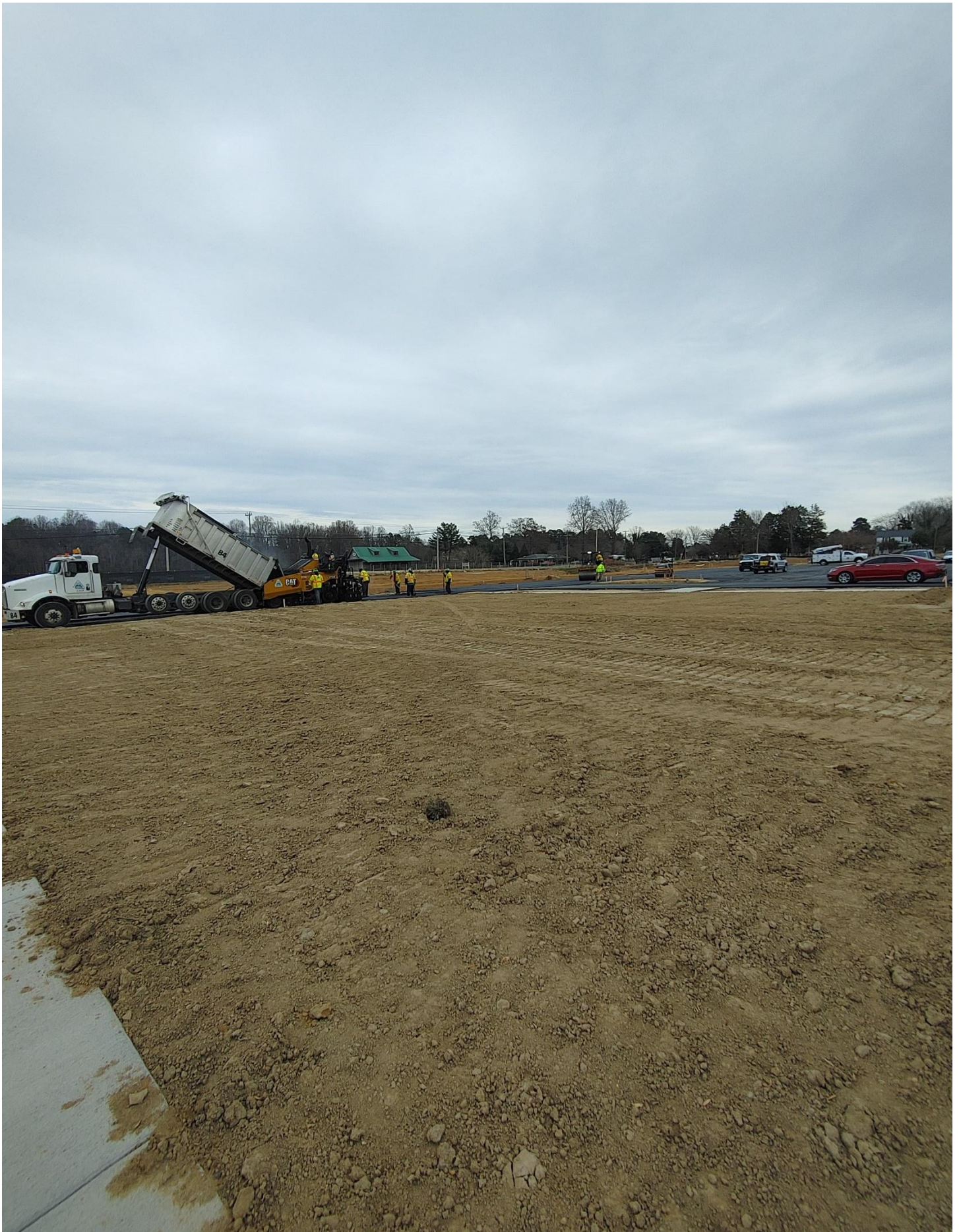
Photo 1 - Asphalt is being laid in the Northeast corner of the Student Parking Lot.
