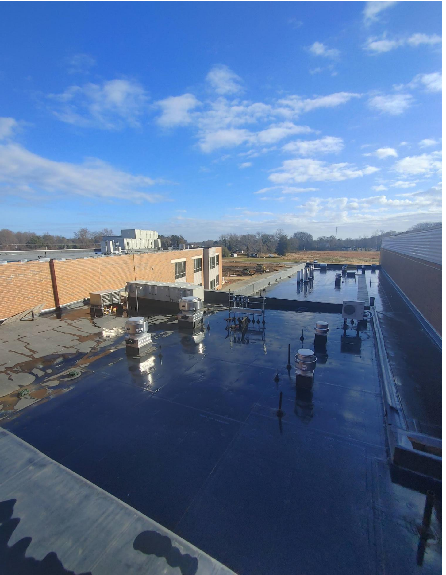
Photo 12 - Roof top units above Kitchen and Mechanical room
